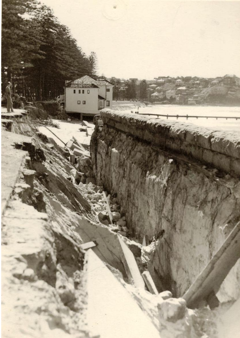
Figure 5.2 North Steyne Collapsed Seawall 27/06/1950
