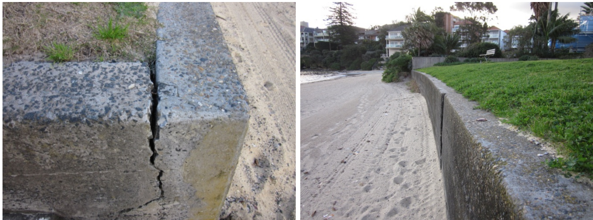
Figure 3.4 Little Manly Seawall Photos of Present Condition
