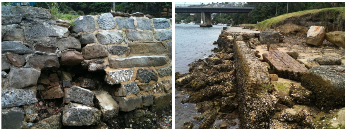
Figure 3.2 Ellery's Punt Reserve Photos of Present Condition
