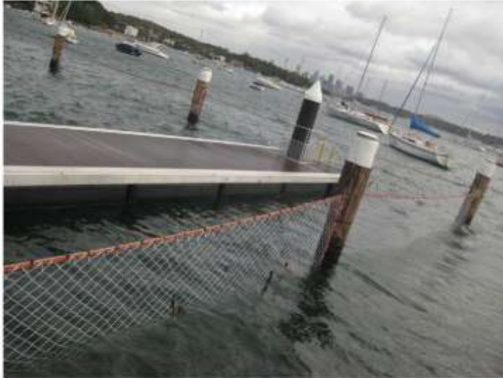
Photograph 1. Trampoline style nets: taught nets suspended on high tension cables and showing attachment to pylons.
